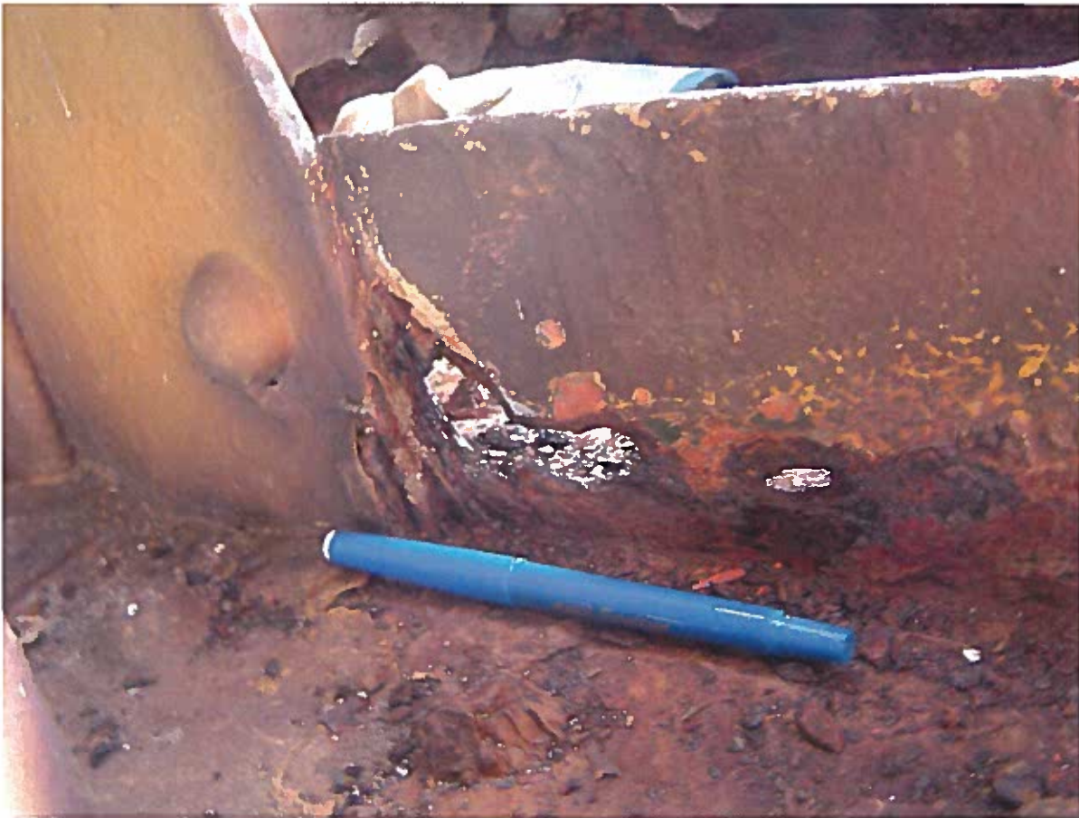
Photo 8: Loss of section in steel superstructure members
