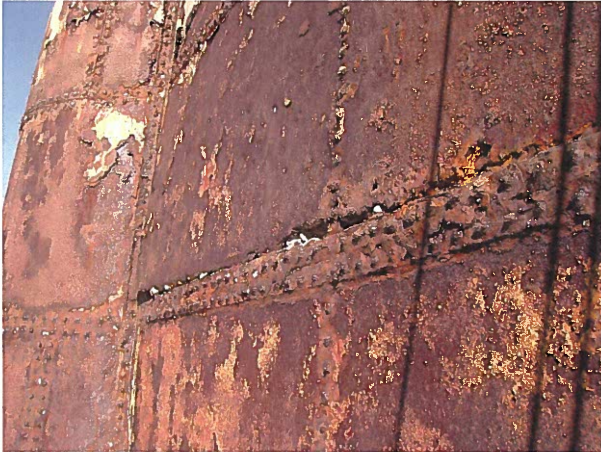
Photo 4: Close up photo at pier cross beam – heavy deterioration of steel shell
