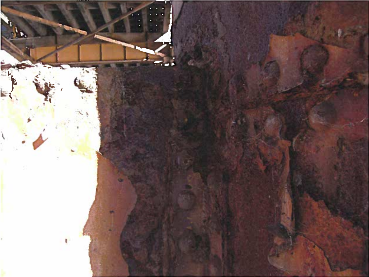
Photo 5: Close-up photo at Pier Cross Beam / Pipe Pier Interface showing loss of steel section and concrete rubble within pipe (heavy deterioration)
