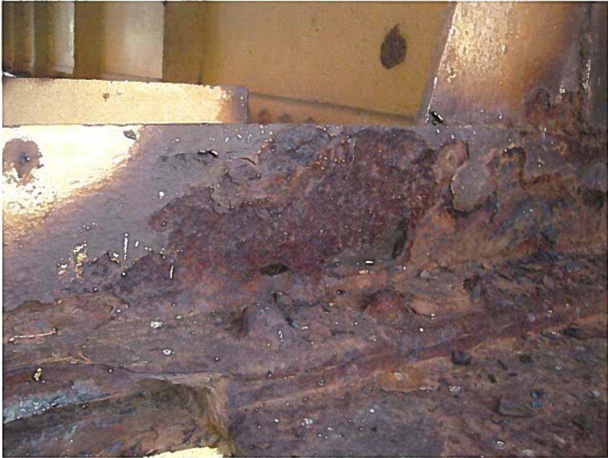
Photo 9: Loss of section in steel superstructure members
