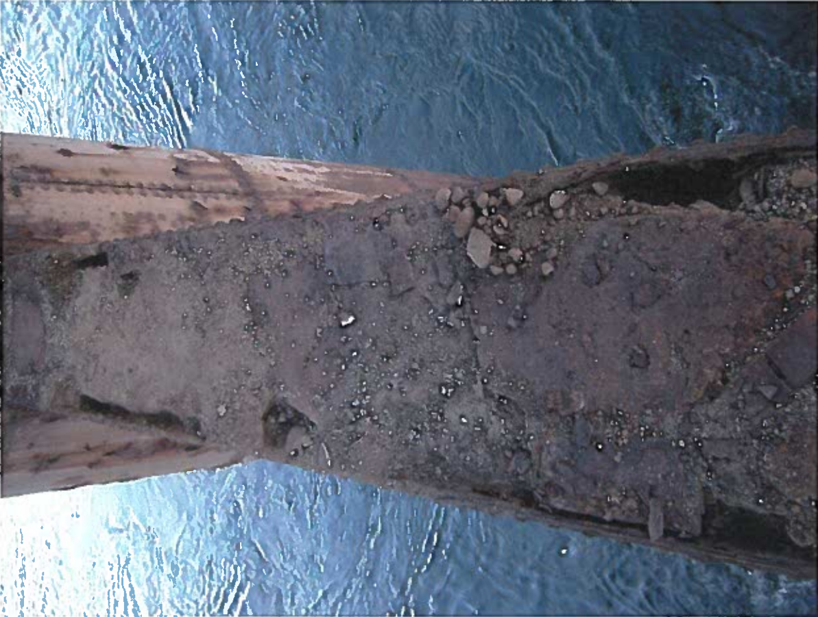
Photo 7: Pier Cross beam showing loss of concrete structure integrity within steel shell
