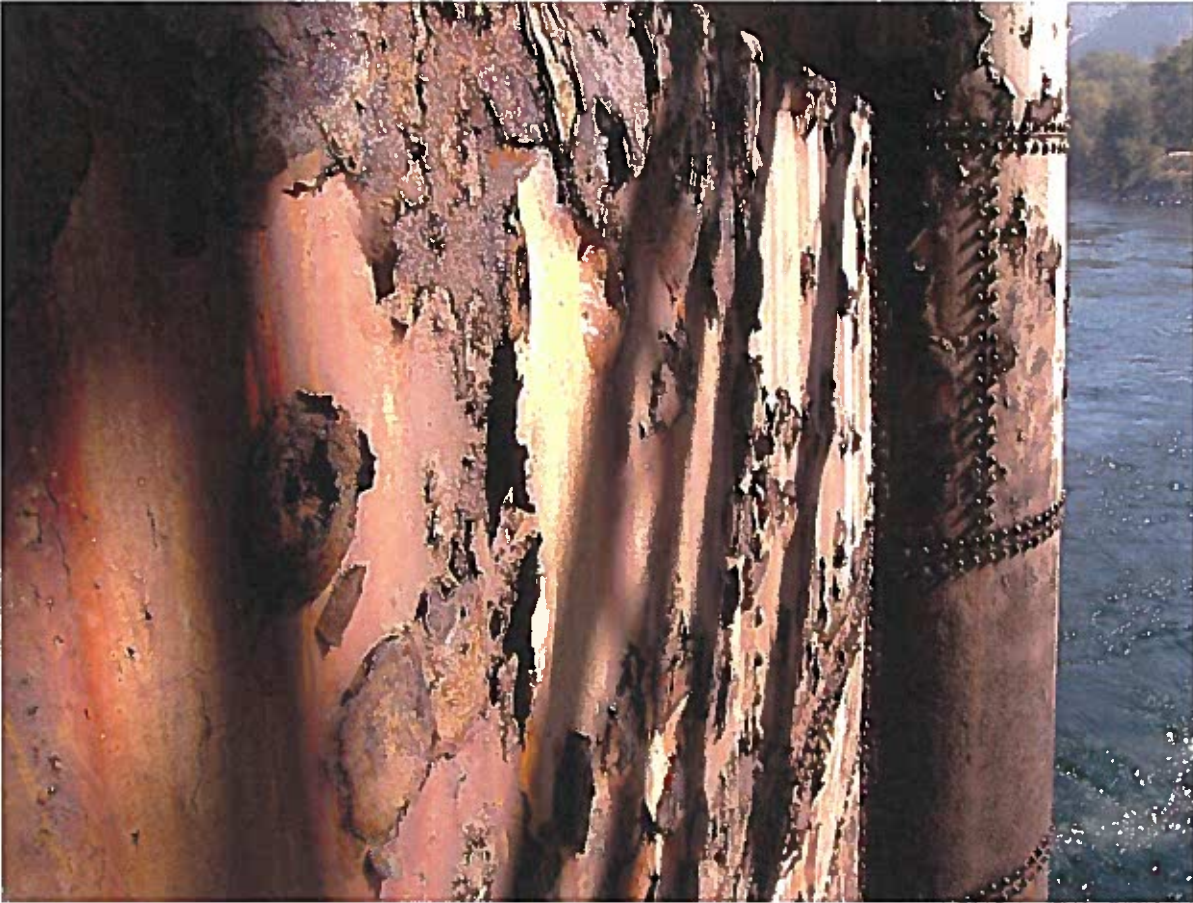
Photo 6: Close up photo at pier cross beam – heavy deterioration of steel shell
