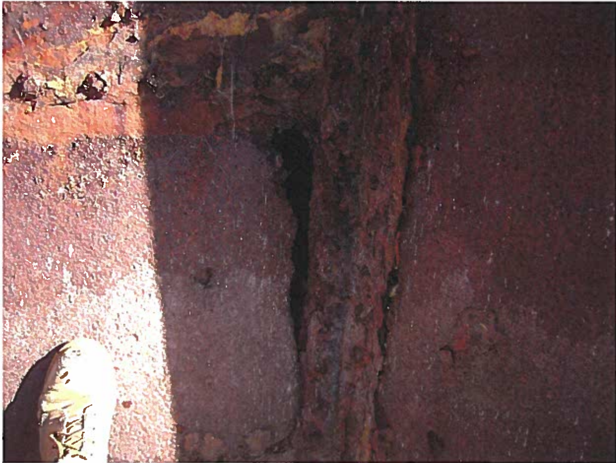
Photo 3: Close up photo at pier cross beam showing loss of concrete structural integrity within steel casing (steel casing can be pushed inwards) and heavy corrosion of the steel shell
