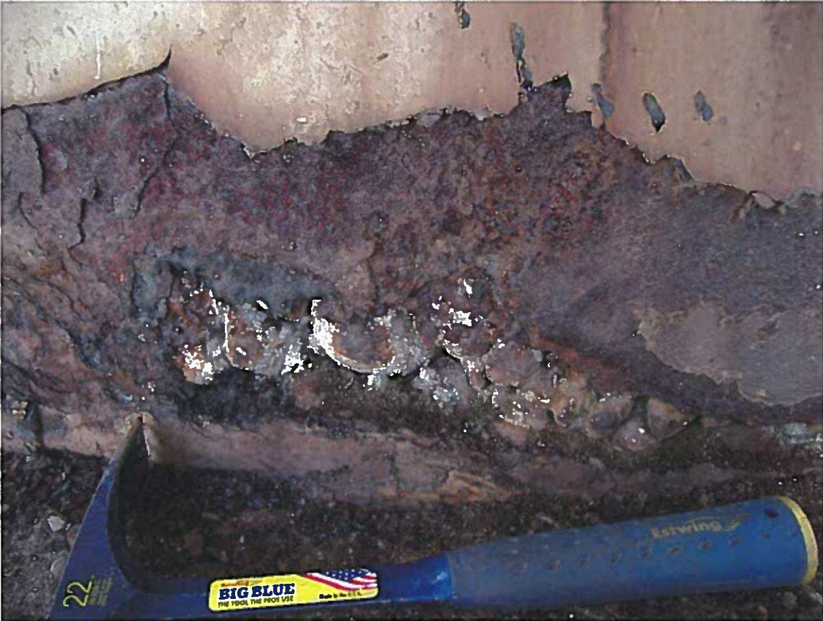
Photo 2: Close-up photo at Pier Cross Beam / Pipe Pier Interface showing loss of steel section and rubble (instead of concretes) within pier legs
