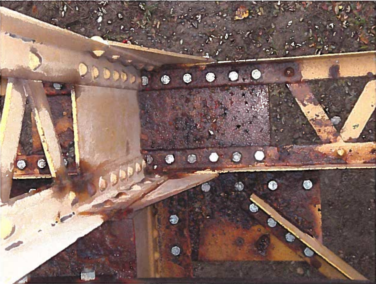
Photo 10: Severe corrosion in steel superstructure connections
