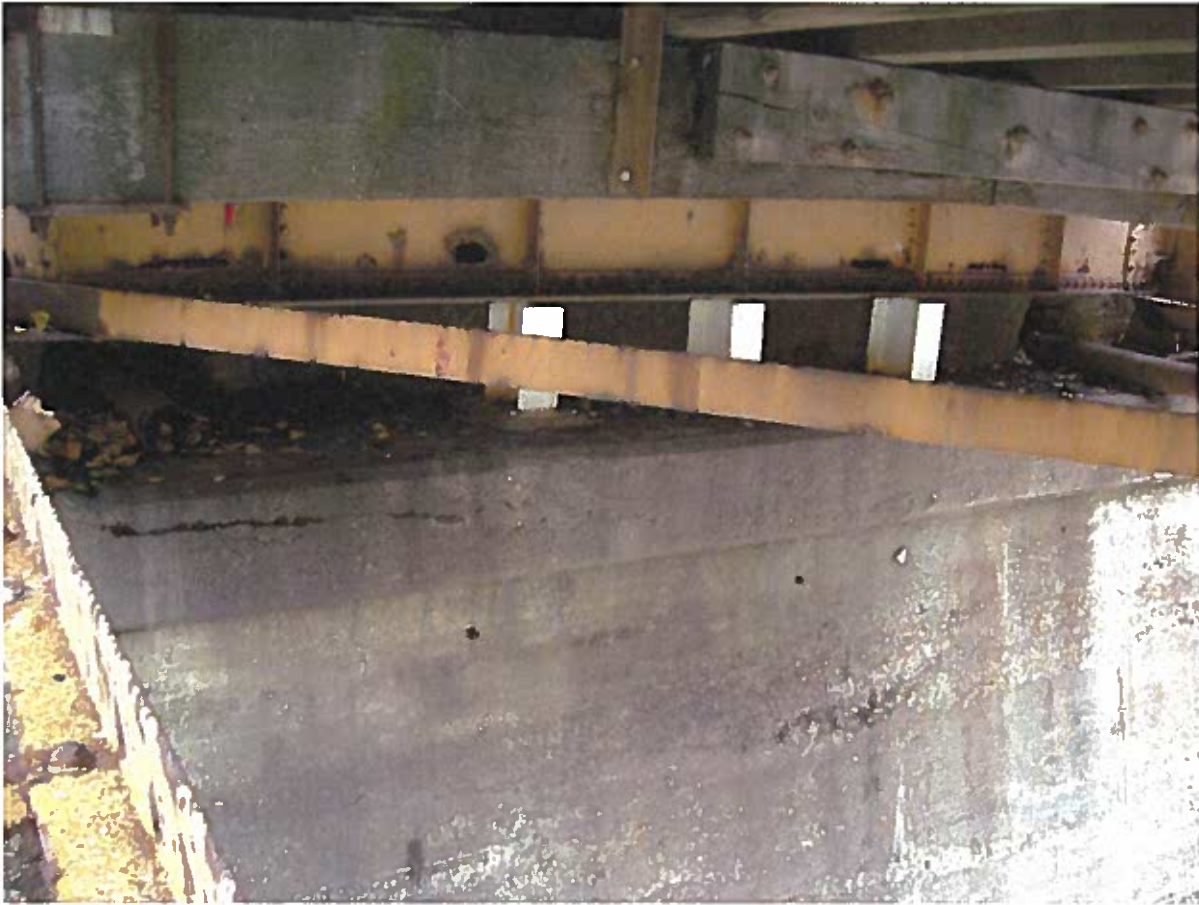
Photo 11: Loss of section in steel superstructure members
